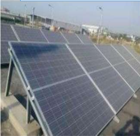
Solar PV - Small capacities in multiple locations
